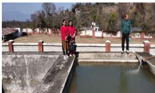
Water storage tank
